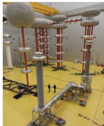
Voltage withstand and bus-charging current switching tests
