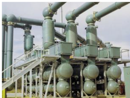
800 kV substation installed in 1979
