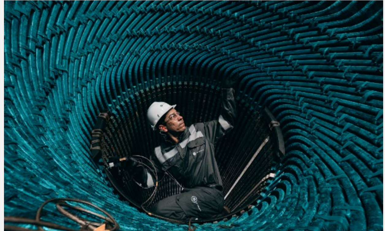
A generator specialist trains at GE Vernova's Houston Learning Center
