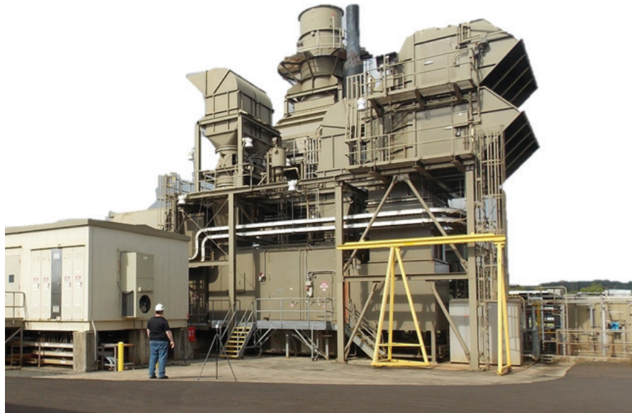
The LM2500 in Combined Cycle on Kauai
