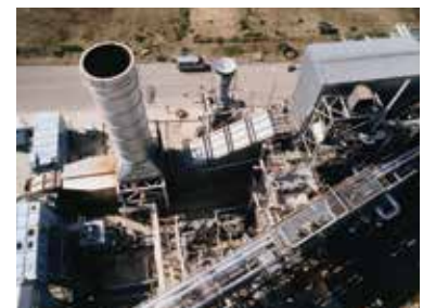
FIGURE 14: High hydrogen fueled 6B.03 gas turbine
