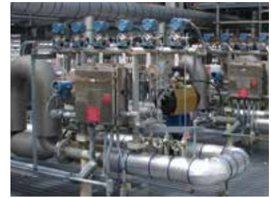
FIGURE 12: Hydrogen/natural gas blending system
