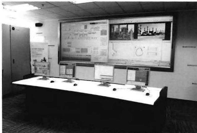
Figure 4 - Automated work station of system operator
