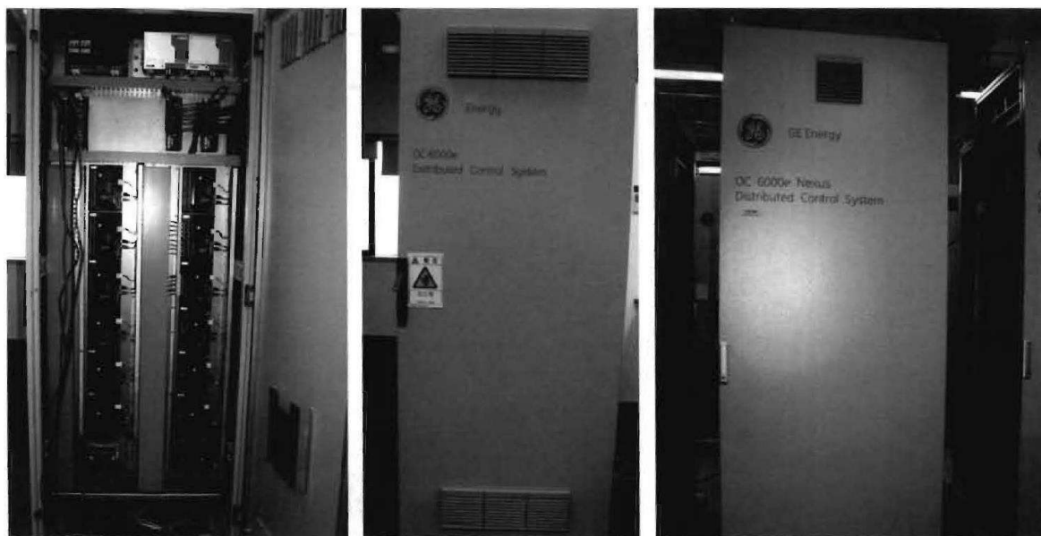
Figure 2 - Exterior of MCC OC 6000e, OC 6000e Nexus instrumental cabinet.
