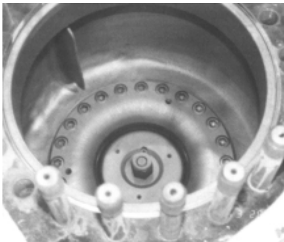
Figure 9. Fayetteville main stream stop/control valve.
