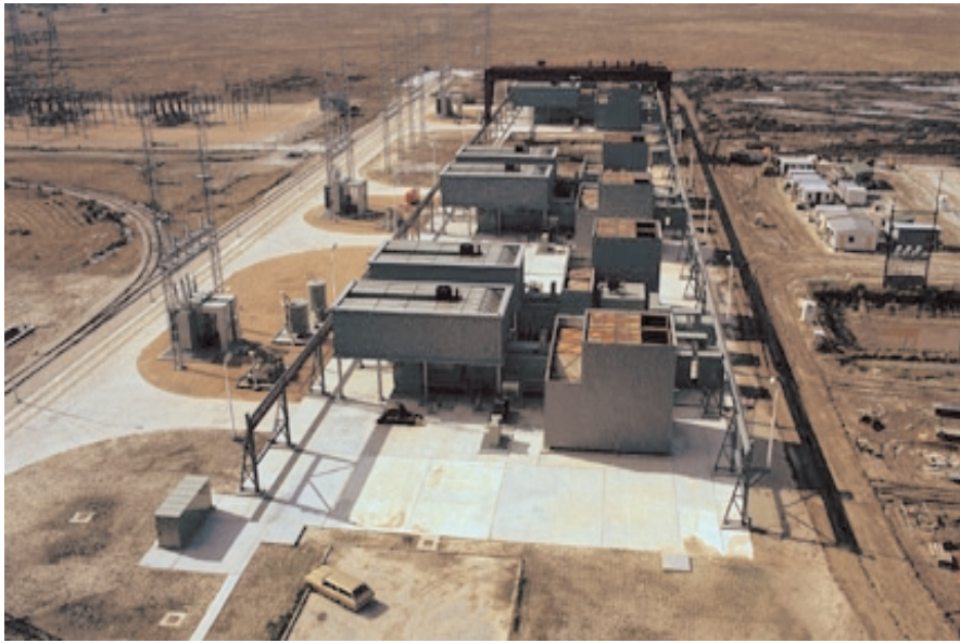
Figure 2. Six MS7001B gas turbines
