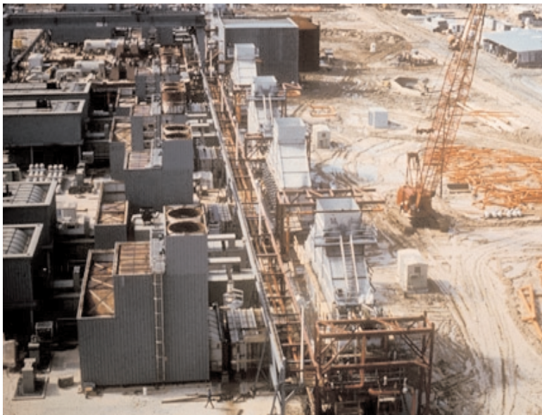
Figure 3. Two STAG 407B combined-cycle steam system installation
