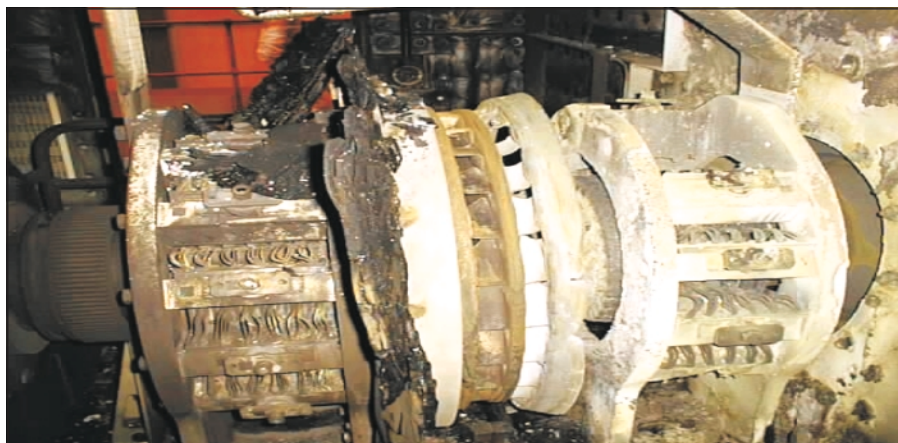
Figure 12. Collector and brush holder neglect
