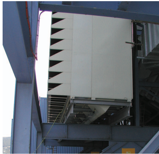
Figure 1. Gas turbine inlet with weather hoods
