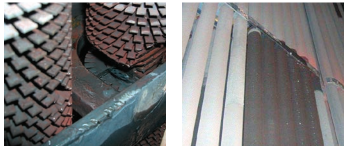
Figure 2: Leaking Tubes from Damaged Restraints
