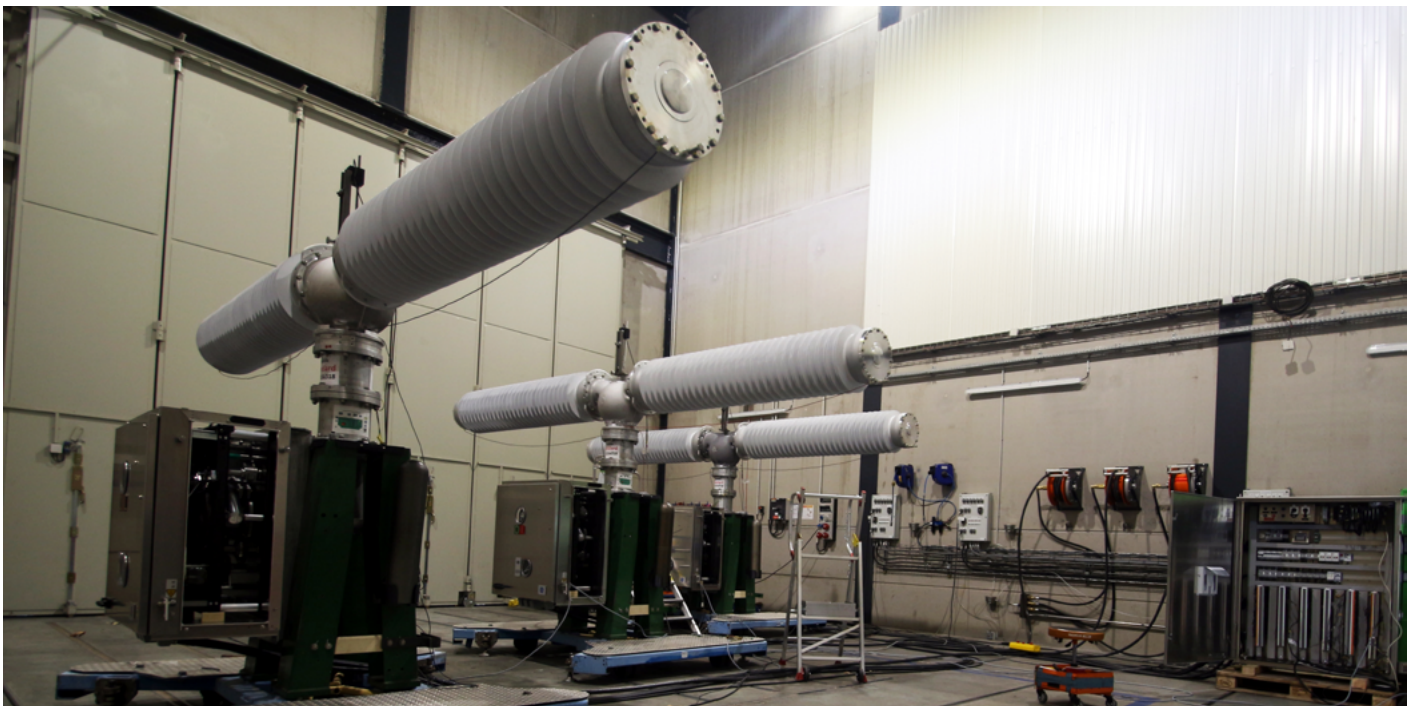
Factory testing of digital native live tank circuit breaker, 3 poles connected to the Low voltage cubicle directly configured and operated with CSD100.
