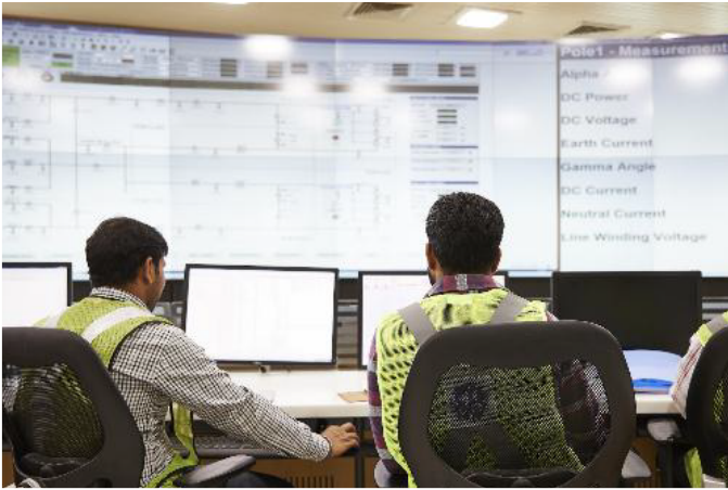
Champa control room
