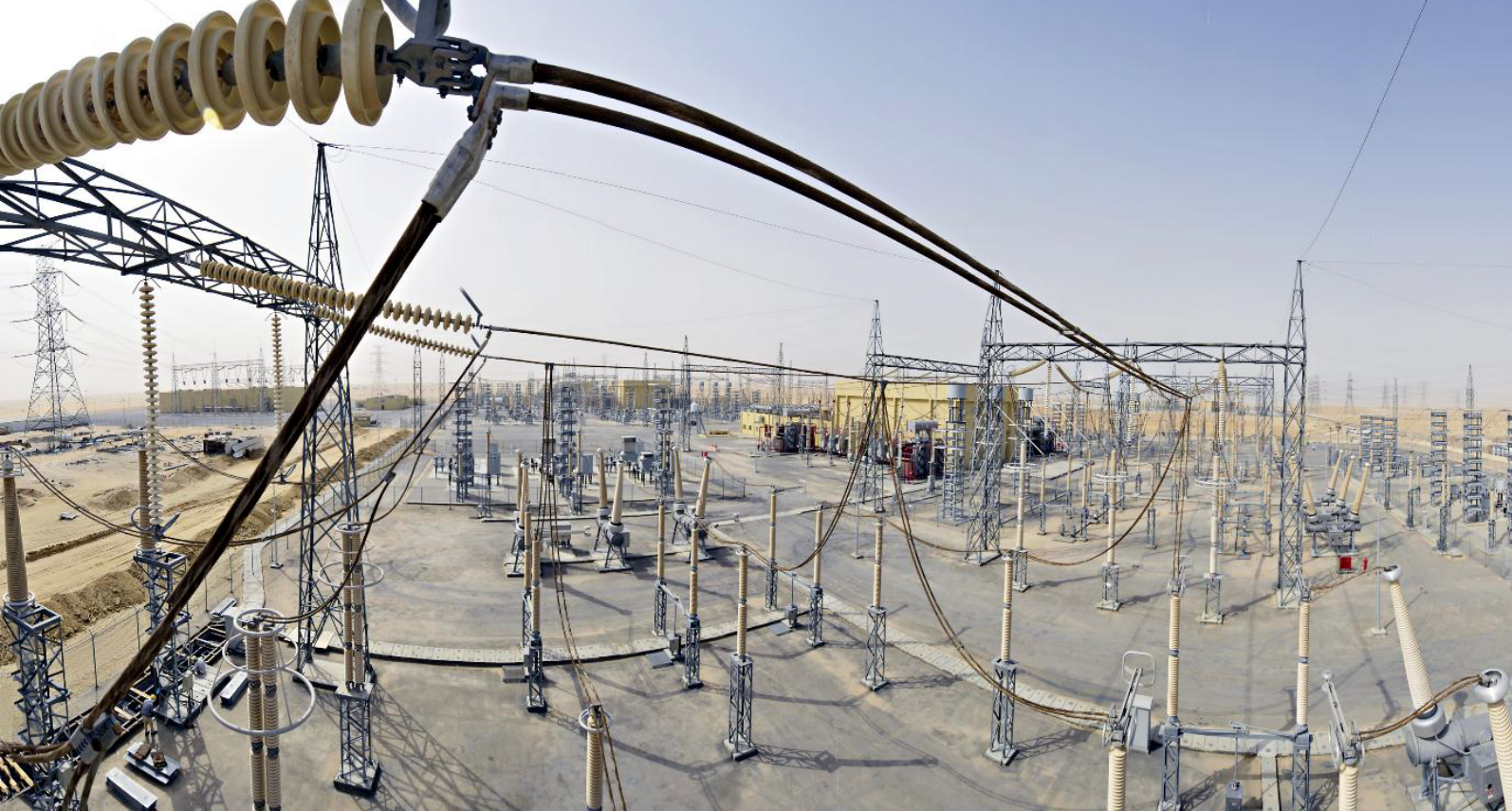
Panorama view of the Fadhili substation
