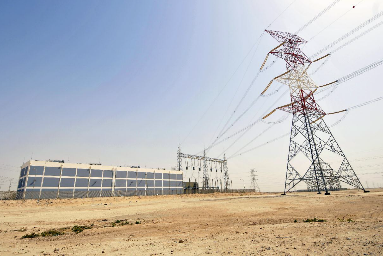
Doha's substation in Qatar
