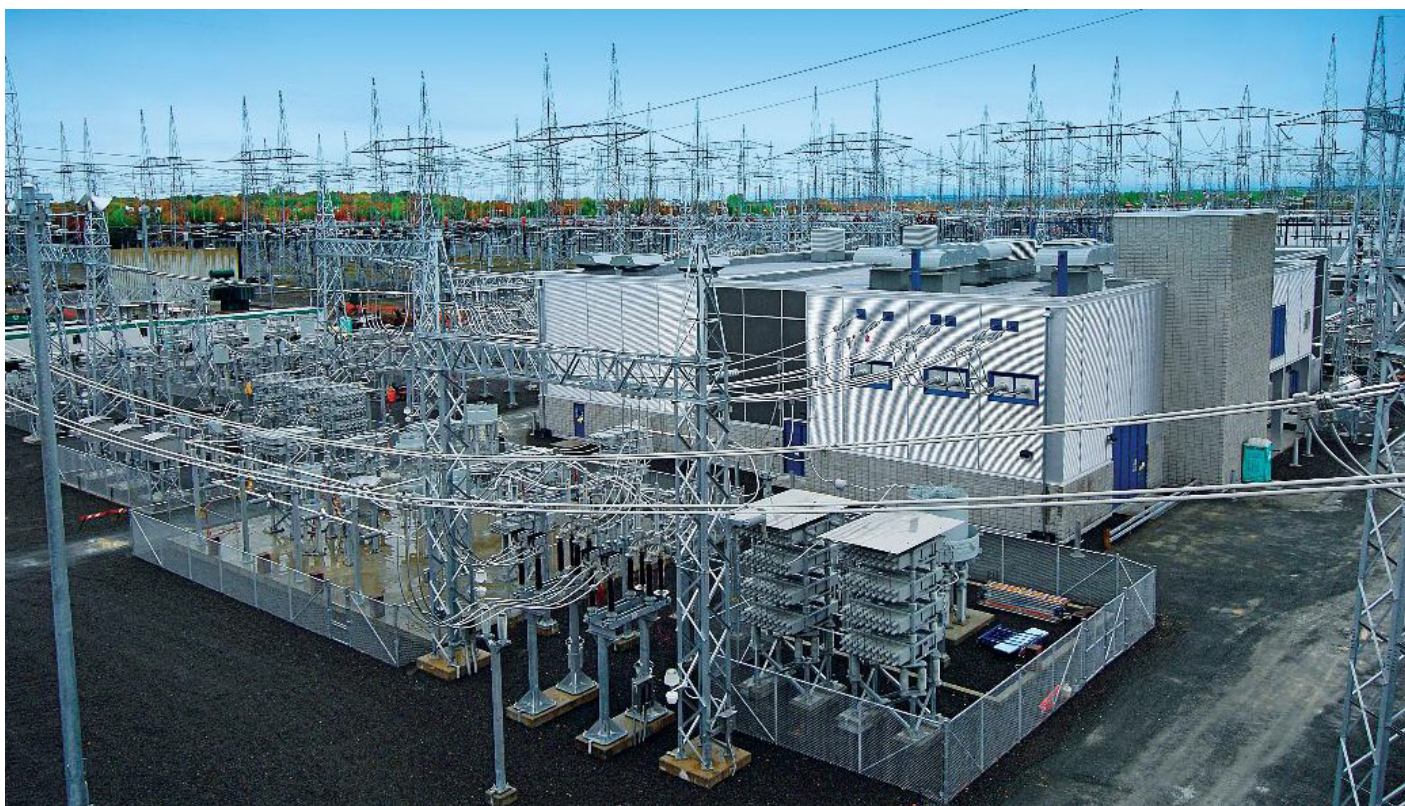
Aerial view of Levis De-icer valve hall and var compensation equipment
