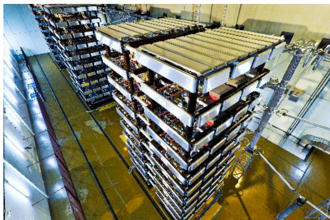
Valve hall after renovation
