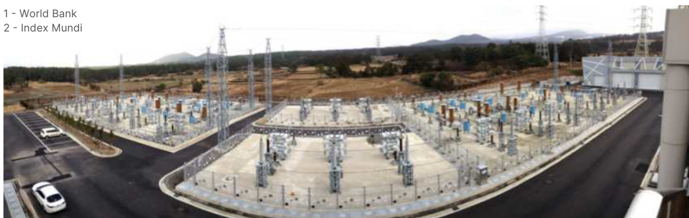
AC filter yard
