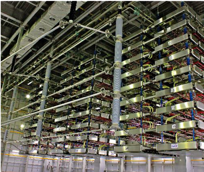
Thyristor valves stack inside the converter hall
