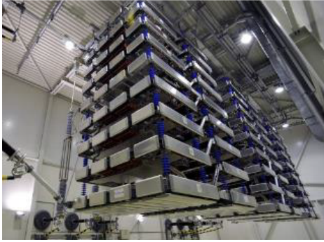
H400 thyristor valves
