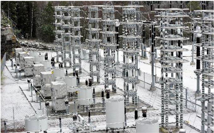
Smoothing reactors and AC Filters
