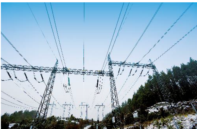
HVDC Line positioned between AC transmission lines
