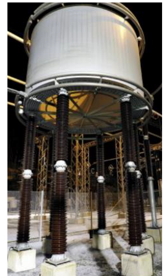
DC Smoothing Reactor
