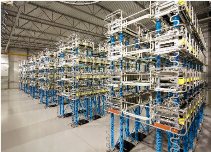
VSC Valves inside the Barkeryd Converter Station Valve Hall
