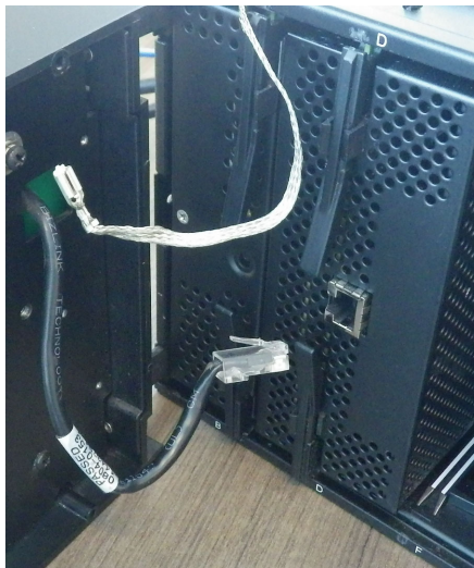
Figure 10-18: Disconnected ground cable and CPU connector
