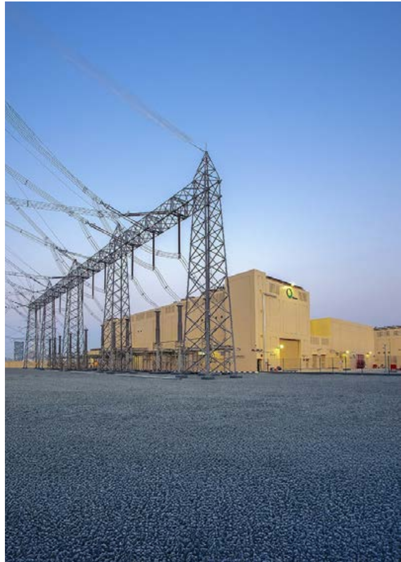
Figure 2. The DEWA Canal Garden Substation, a 400/132 kV facility in Dubai's Discovery Garden area, was built for Dubai Expo 2020. With a capacity of 2000 MVA, it eases load on nearby areas and supports future growth. GE Vernova led the project, with Aztec Middle East handling civil works. Managed by DEWA, the substation aligns with DEWA's clean energy strategy, incorporating advanced grid technologies to drive Dubai's transition to a sustainable energy future.
