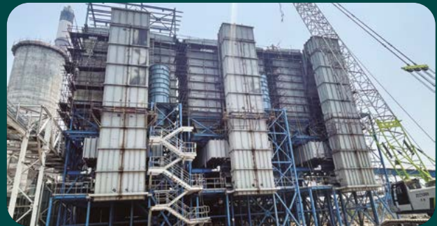
↗ Air Quality Control Systems
