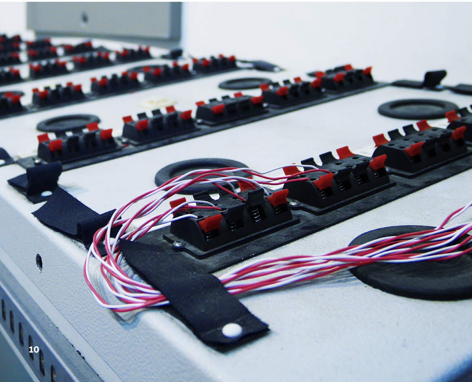
View of temperature sensors control panel inside temperature rise testing room
