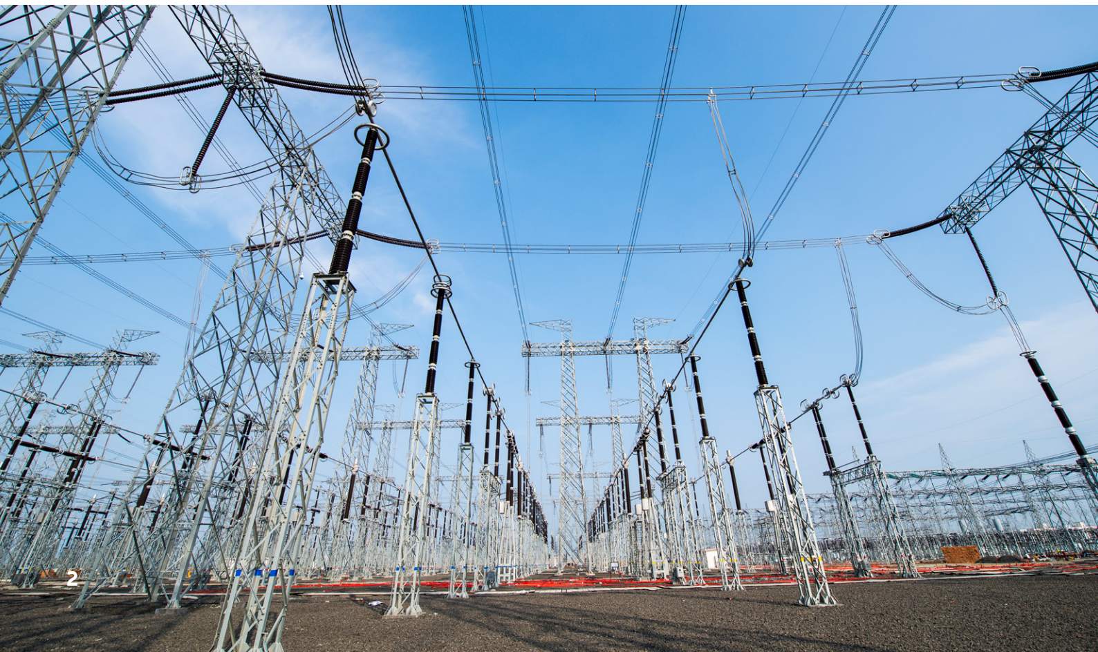
View of a High Voltage substation
