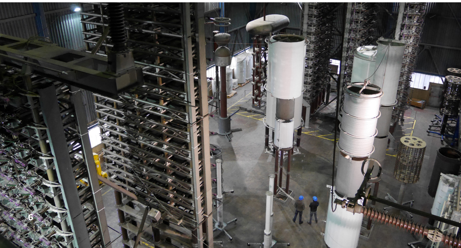
Top view of High Power Test Laboratory Synthetic lab. Capacitor bank (left) and reactor bank (center, white)
