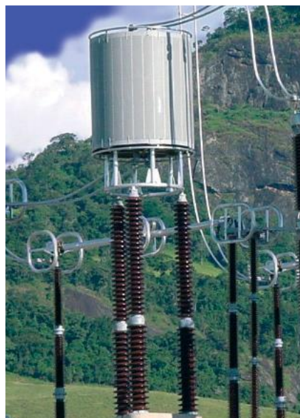
Vertical pedestal A line trap mounted on CCVT
