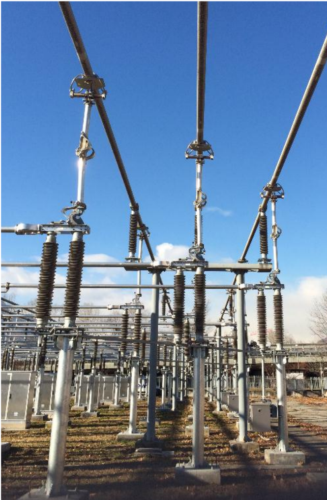
SPVL disconnecter type with DWatch mechanism installed
