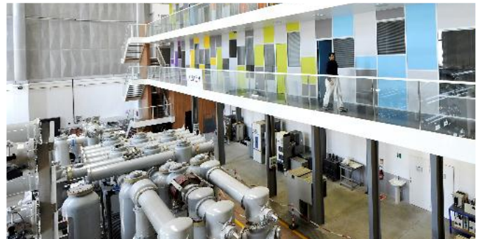
Real equipment accessible at GE Training Centers
