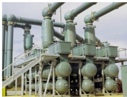
800 kV substation installed in 1979
