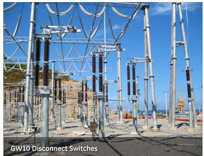
GW10 Disconnect Switches
