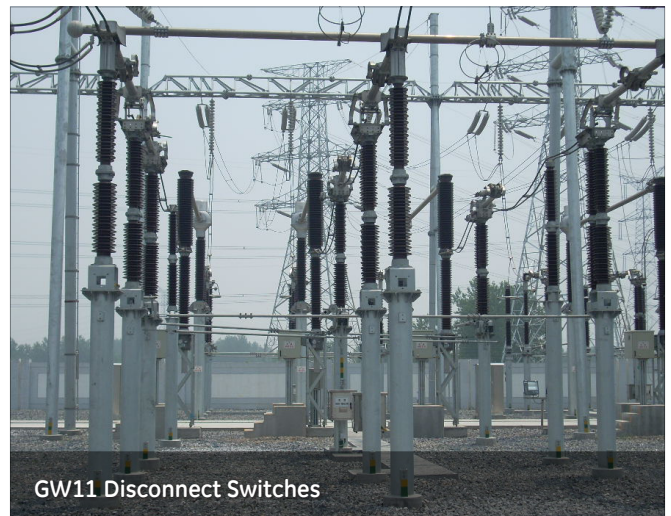
GW11 Disconnect Switches
