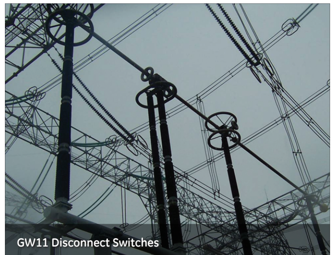
GW11 Disconnect Switches
