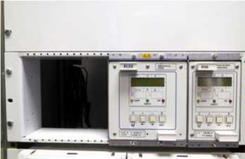
Typical relay panel with KCEG and KCGG Relays
