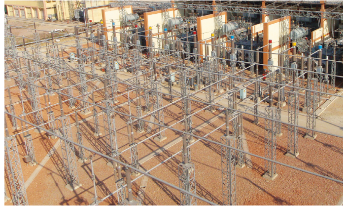
Typical AIS installation
