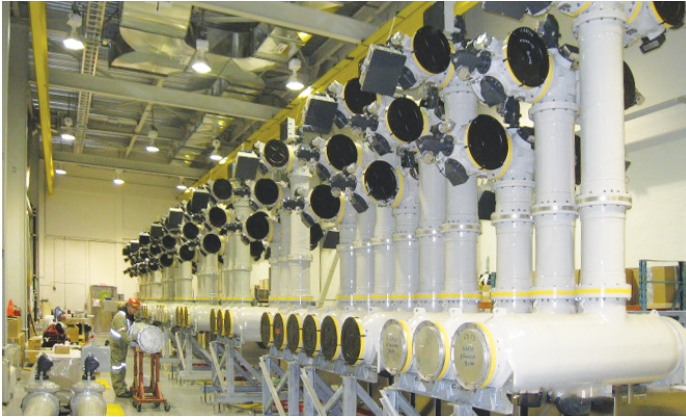
Typical GIS installation
