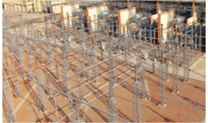
Typical AIS installation
