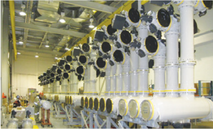
Typical GIS installation
