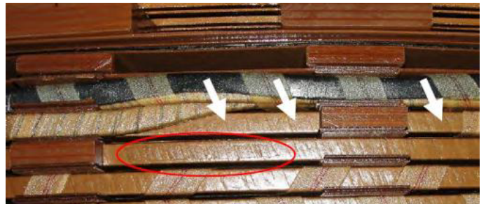
Figure 3: Paper sampling locations must be chosen according to the accessibility and rebuilt feasibility. Locations should be reasonably representative of winding temperature conditions or hot spot conditions.
