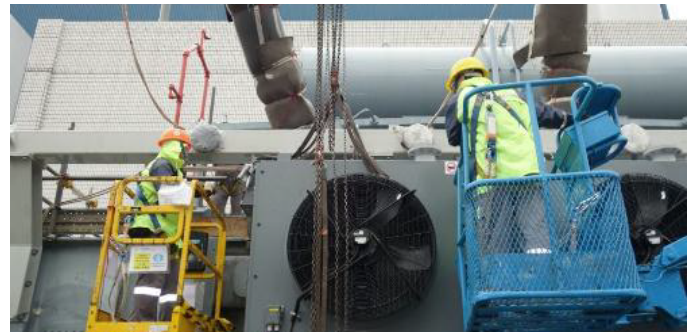
Figure 4: Improving cooling efficiency with upgrade of coolers and control cubicles on a 23 kV/435 kV three phases 420 MVA generator step up transformer.
