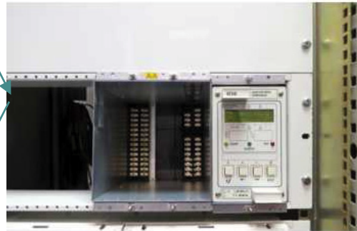
Withdraw the KCEG relay
