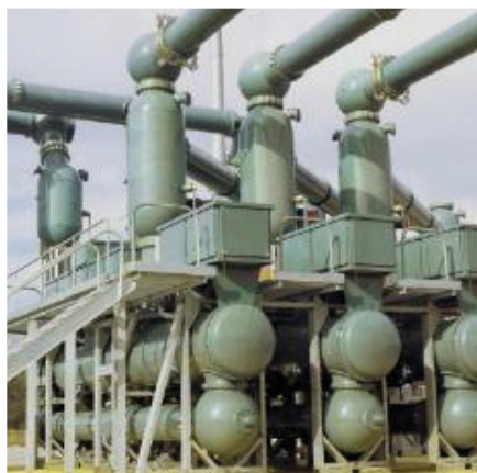
800 kV substation installed in 1979
