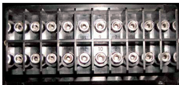
FT switch terminals 1 thru 20 (rear view)
