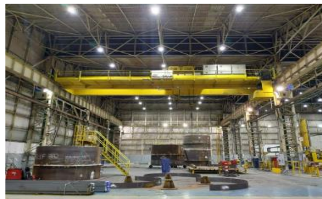
Replacement of USP and CASLSP lighting by LED on Taubate GE Hydro site (2021)
