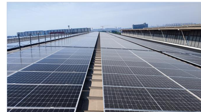
Solar roof made of 13 000 solar panels installed at GE Hydro Tianjin site
