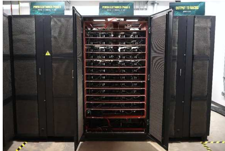
GE Vernova's solid-state transformer prototype at our lab in Malta, New York.
