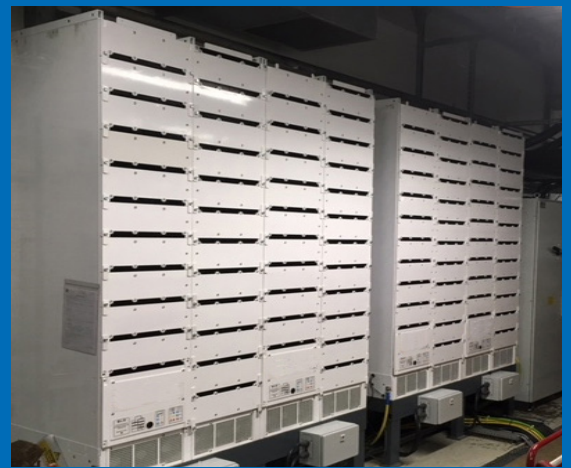
1MW Battery Under Integrated System Test at the Marine Power Test Facility, UK.
