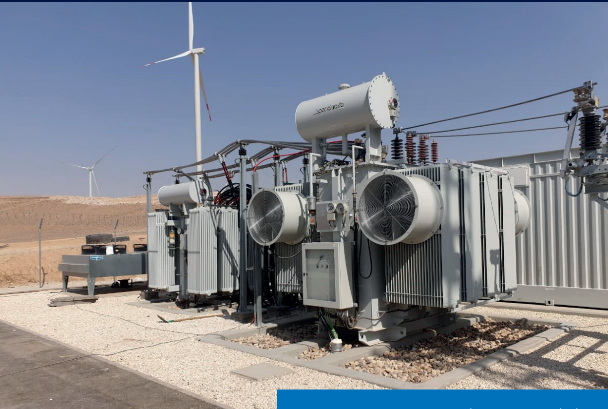
Power Conversion equipment on site at the Mass Energy Wind Farm
