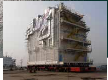
FPSO for Libra Field e-House electrical distribution module being installed on FPSO topside
