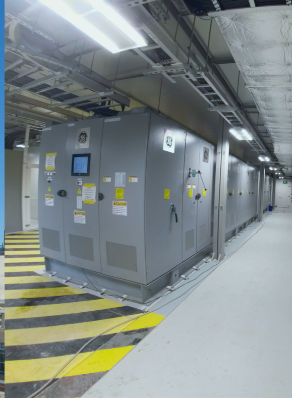
Inside an e-house
