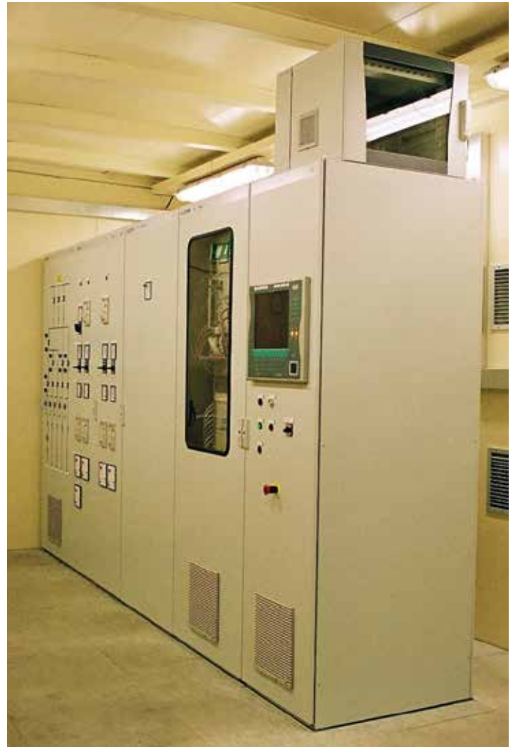
Closed-loop control, open-loop control and protection cubicles of the dynamic compensation
