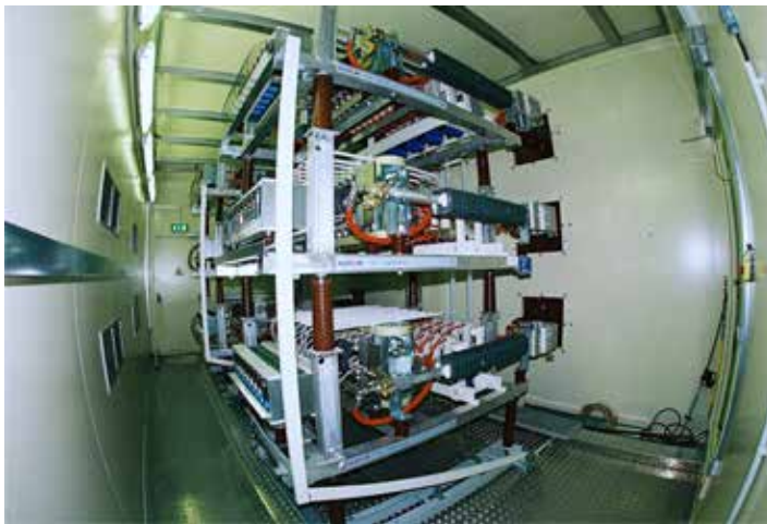
Two phase racks of the 250 Mvar thyristor converter connected in series in the sheet steel container
