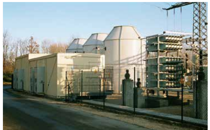
One phase of the capacitor bank of the 100 Hz filter circuit with twin bridge comparison protection, anti-noise enclosures of the self-cooling TCR reactors, and the laminate sheet steel container for the converter and closed-loop control.
