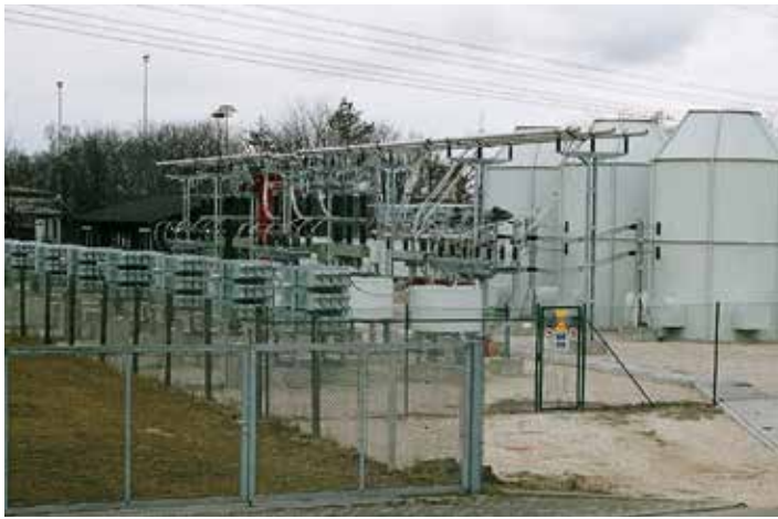
The outdoor switchgear of the 67m long and 31m wide dynamic compensation looking from East to West.
