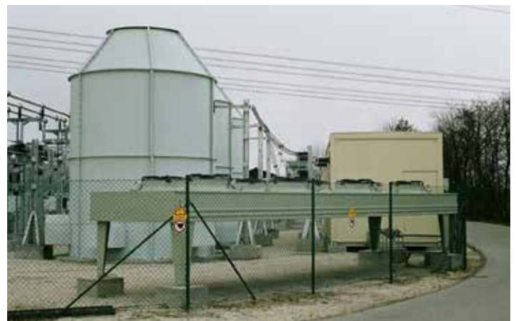
Anti-noise enclosures of the self-cooling TCR reactors; on the right, sheet steel container of laminate design; in the foreground, the glycol water/air heat exchanger of the thyristor controller.
