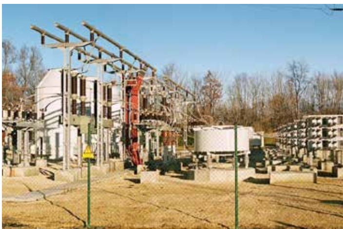
The noise-insulated TCR reactors are clearly visible, as well as the container for the converter and closed-loop control, and the 33 kV aluminium tubing busbar.
