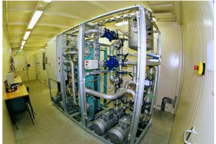
Cooling system of the converter in the sheet steel container. Control valve in the glycol water circuit for continuous adjustment of treated water temperature as a function of ambient temperature. Twin pumps. In the background is the closed-loop control of the dynamic compensation.
