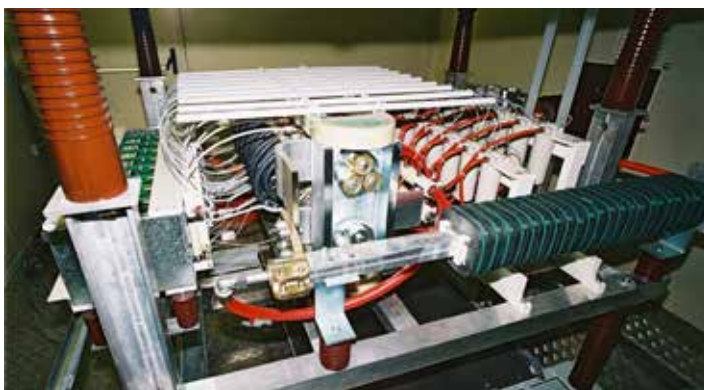
Valve platform with water-cooled thyristor twin column, water-cooled RCattenuation and water-cooled ferrite core reactors
