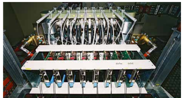
Twin column with water-cooled 100 mm disc thyristors. In the foreground are the thyristor section electronics for control and monitoring via synthetic optical fibres.
