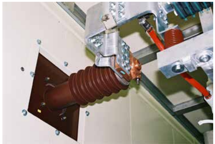
Power supply connection for 4000 A from the insulating bushing to the thyristor rack
