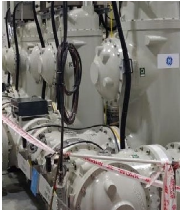
GIS bays for Bhutan Power Corporation at Dochula
