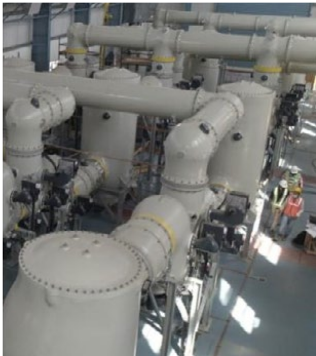
PGCIL, Phagi, Rajasthan First GE Make 765KV GIS
