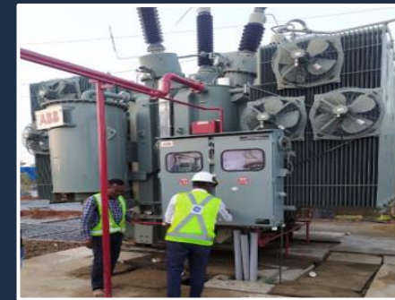
21.6 MVA, 132/27kV TSS Transformer commissioned for National Mineral Development Corporation at Nagarnar
