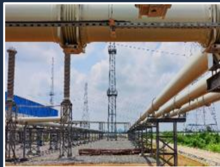
Eighteen bays of 400 kV GIS with 3600 meters Gas Insulated Busbar for L&T at Thallayapalem in Andhra Pradesh
