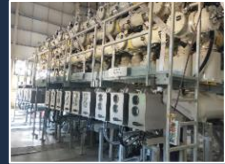
220 kV bay along with 220/34.5 KV, 50 MVA Transformer commissioned at NTPC Unchahar
