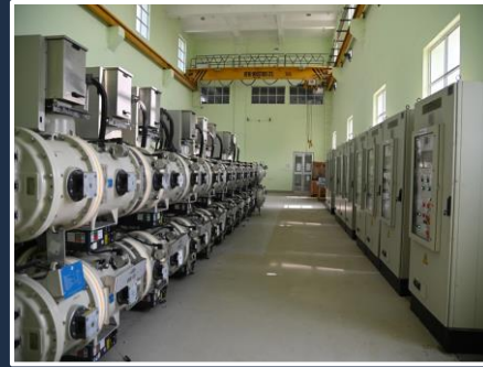
132 kV GIS at Ramnagar for West Bengal State Electricity Transmission Company Limited
