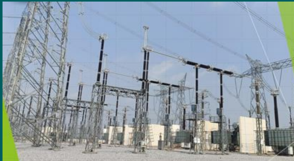
765kV AIS Substation at Adani Warangal
