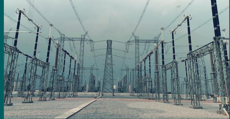
765kV AIS Substation at Adani C'peta
