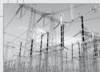
765 kV Anta substation in Rajasthan successfully commissioned by Alstom
