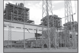
3x660 MW e-BoP project at Lalitpur thermal power plant for Bajaj Infrastructure Limited
