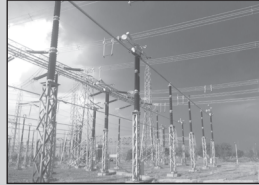
400 kV AIS substation at Amreli for GETCO
