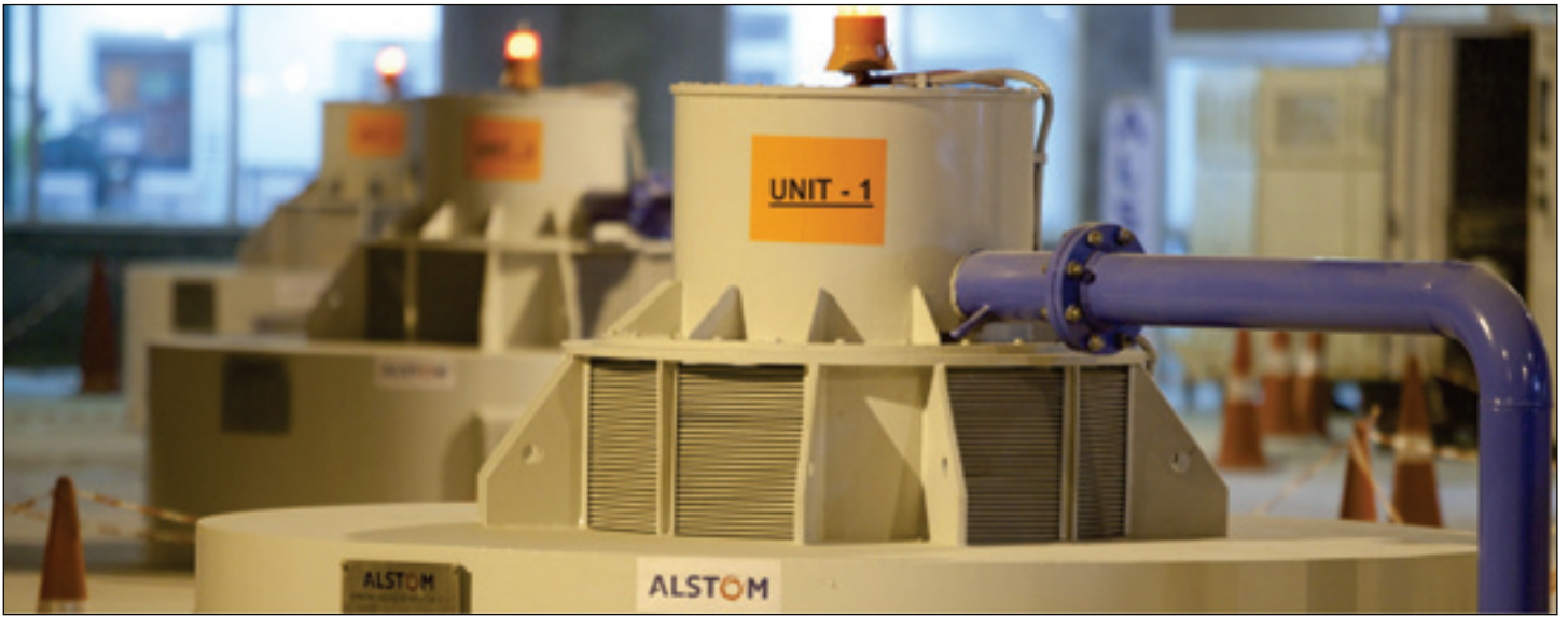
3x77 MW Chamera III Hydro Electric Project successfully commissioned by Alstom
