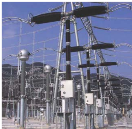
India's first 765 kV substation at NTPC's Sipat Power Plant commissioned by ALSTOM T&D India
