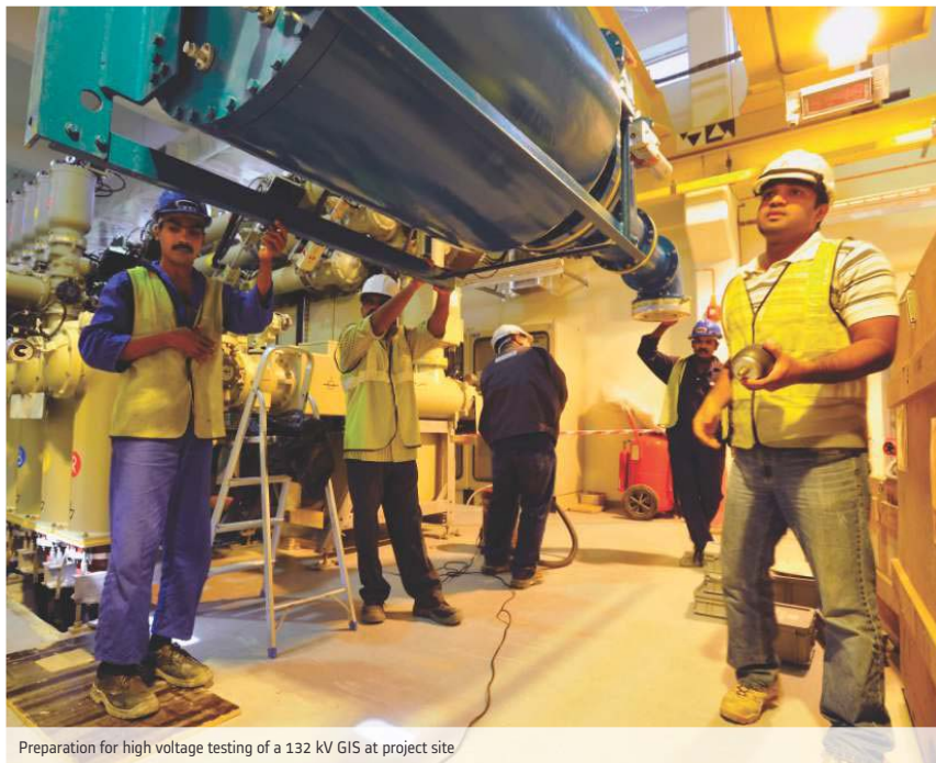
Preparation for high voltage testing of a 132 kV GIS at project site
